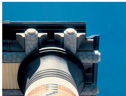
The same off-the peg 'rilled plank' architectural element on another JOA building - and with a smaller budget.
